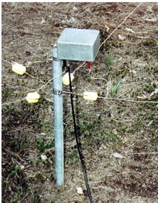
Figure 4—A photo of the central connection point at the base of a two-loop system, as installed at K9AY.
